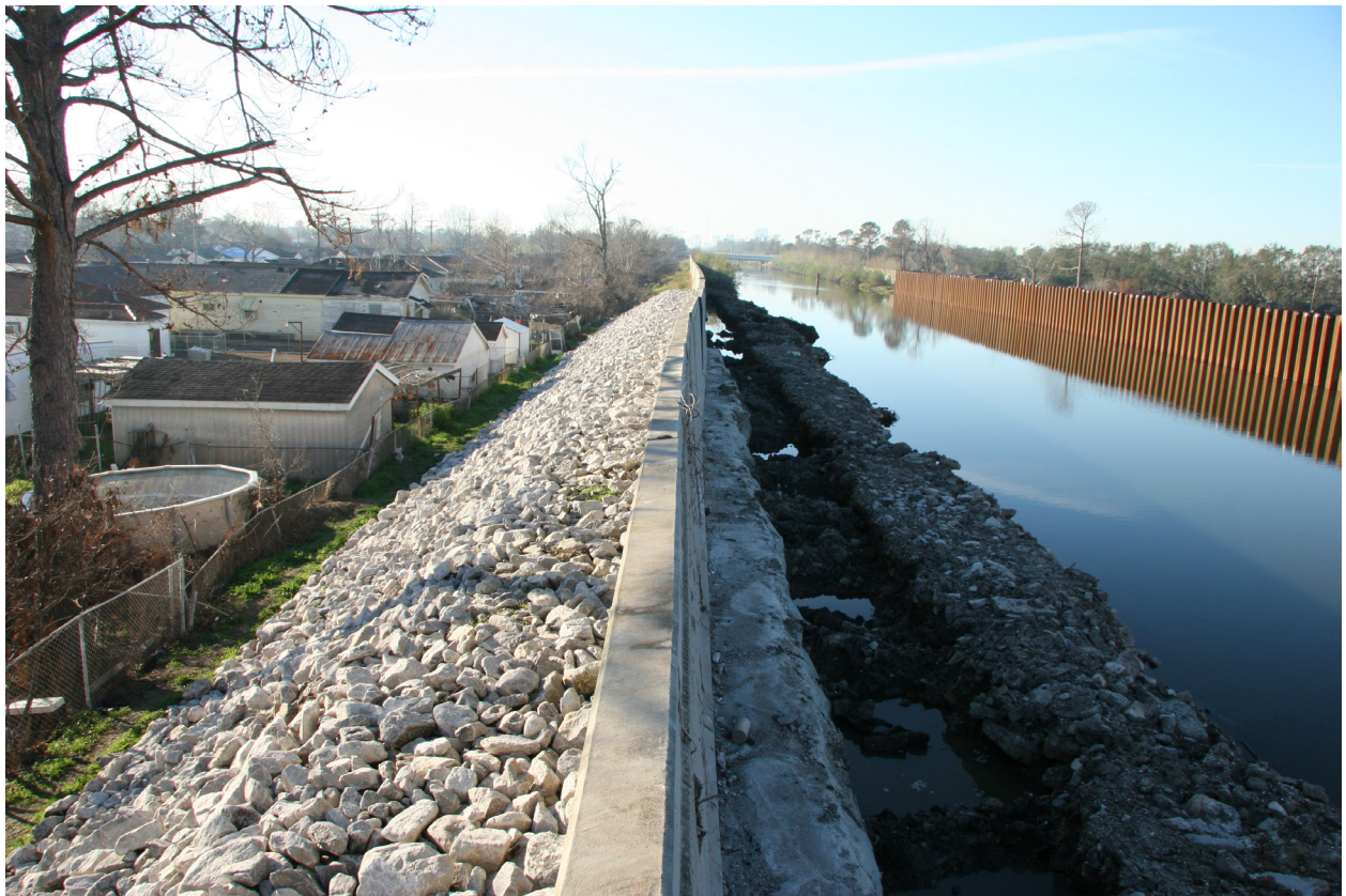
FIGURE 3: VIEW ALONG THE EAST SIDE OF THE LONDON AVENUE CANAL NEAR ROBERT E. LEE BOULEVARD SHOWING THE ENCROACHMENT OF HOMES AGAINST THE SLOPE OF THE LEVEE, A SITUATION COMMON ACROSS NEW ORLEANS. 6
